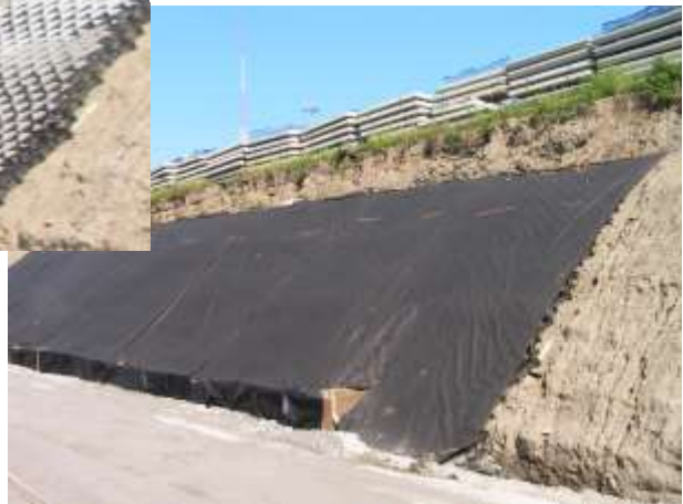
Below: Completed Installation with Geotextile Cover – For Protection Prior to Backfill of Slope
