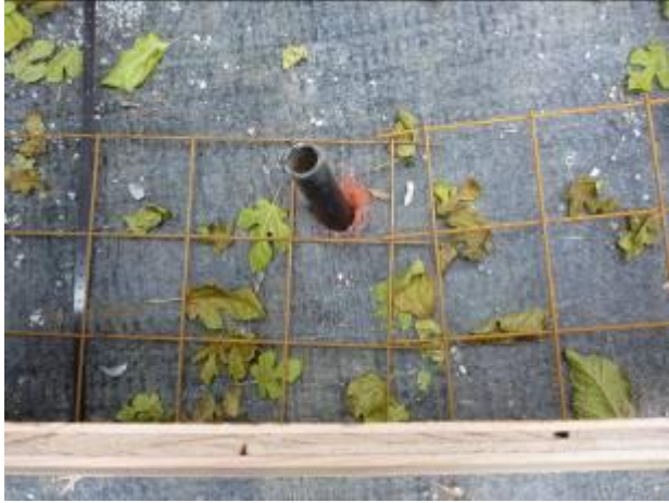
Pipes installed within the anchor strip form along the Steepest section of the slope.
