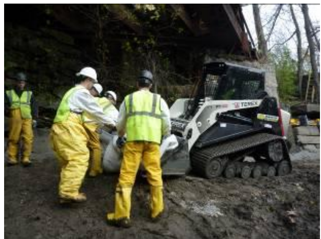
On the upstream end of the canal, a bobcat was used to transport materials.
