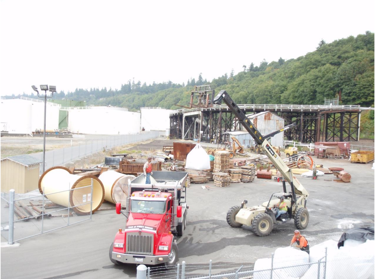
Loading AquaBlok from site delivered bulk bags into aggregate truck with stone slinger
